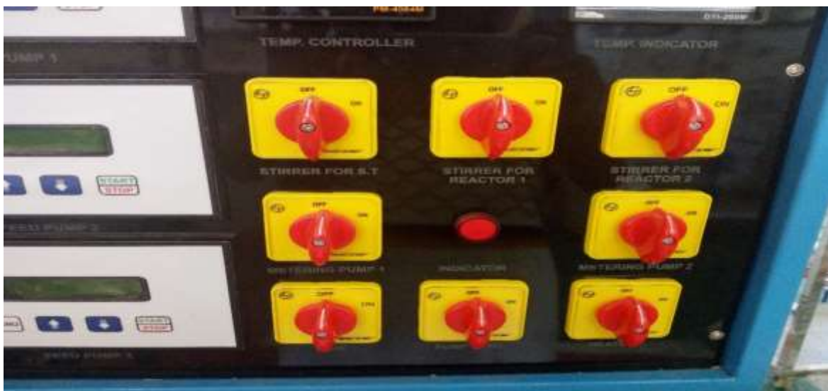
Figure (3.5): Control panel
