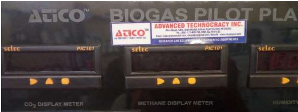
Figure (3.4): Control panel
