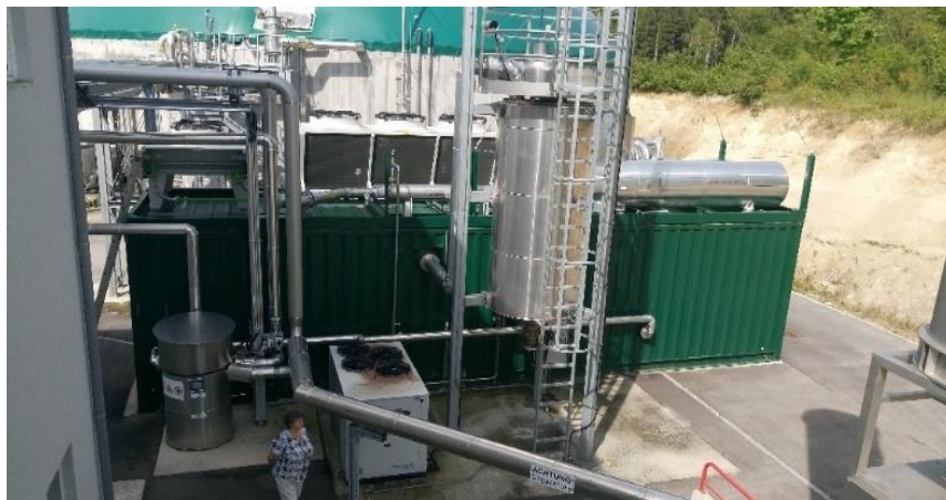
Figure 3. 9: Electricity generator box
