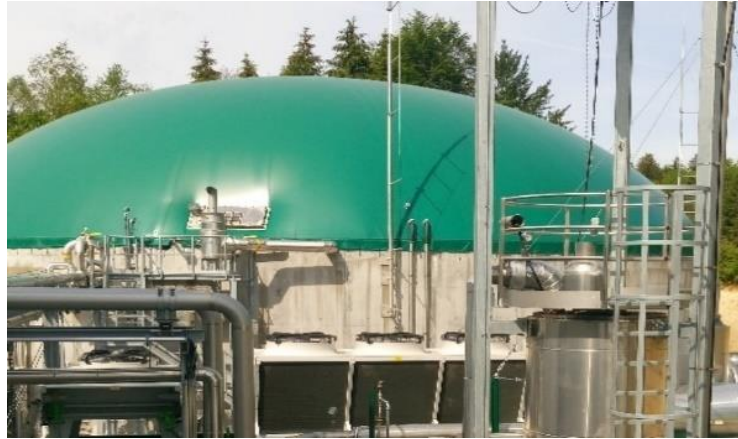
Figure 3. 8: Liquid effluent storage tank
