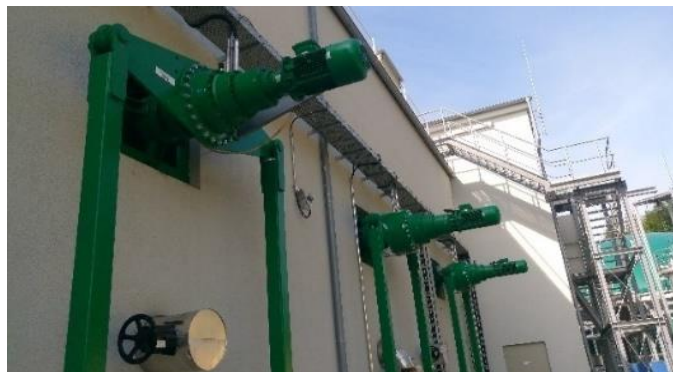
Figure 3. 5: Slurry mixing system
