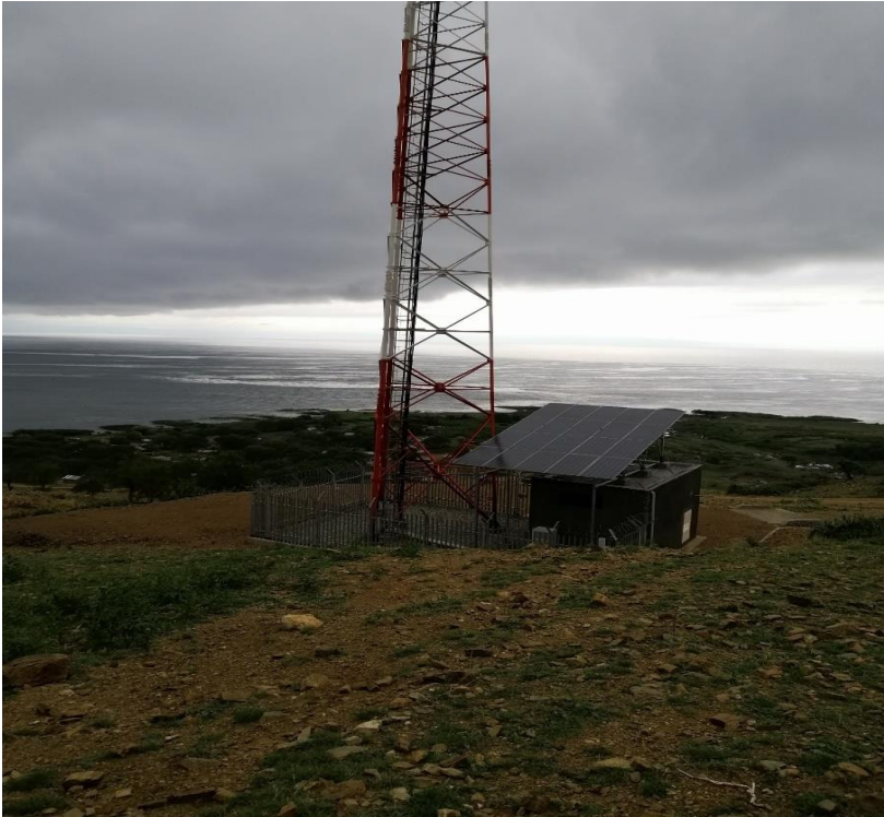
Photo Plate 4: A solar powered telecommunication mast at Kibiro in Kigorobya Sub-county, Hoima.
