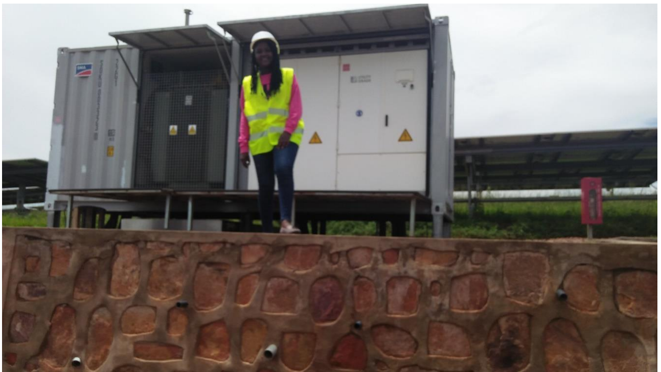
One of the converter At globalwatt solar power plant in Rwamagana district
