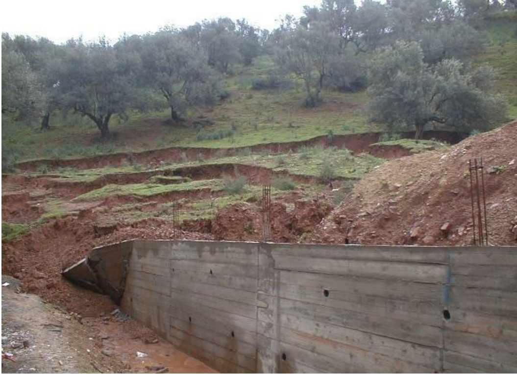
Figure 2.11 : Landslide at Beni Amrane , Department of Boumerdes, causing damage to retaining wall, January 2003(Salah-Mars et al.2004).
