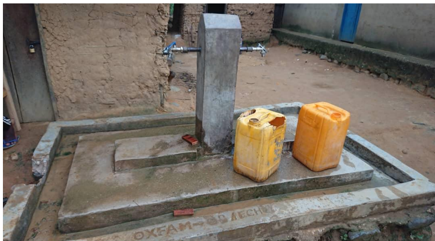
Figure 14: A water hydrant built by OXFAM in Kitutu locality.
