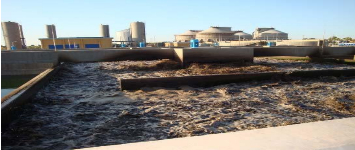
Figure 3. 5: the Aeration tank (Activated sludge)
