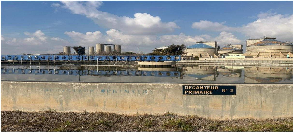
Figure 3. 4: The primary clarifier
