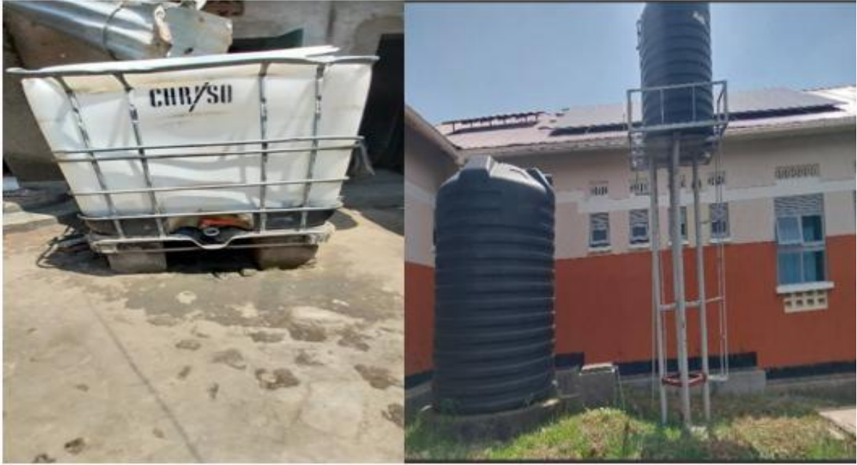
Plate 1.3.3: The Rainwater Harvest tanks are installed in household & institutions' buildings Source: (Author's Work, 2025)
