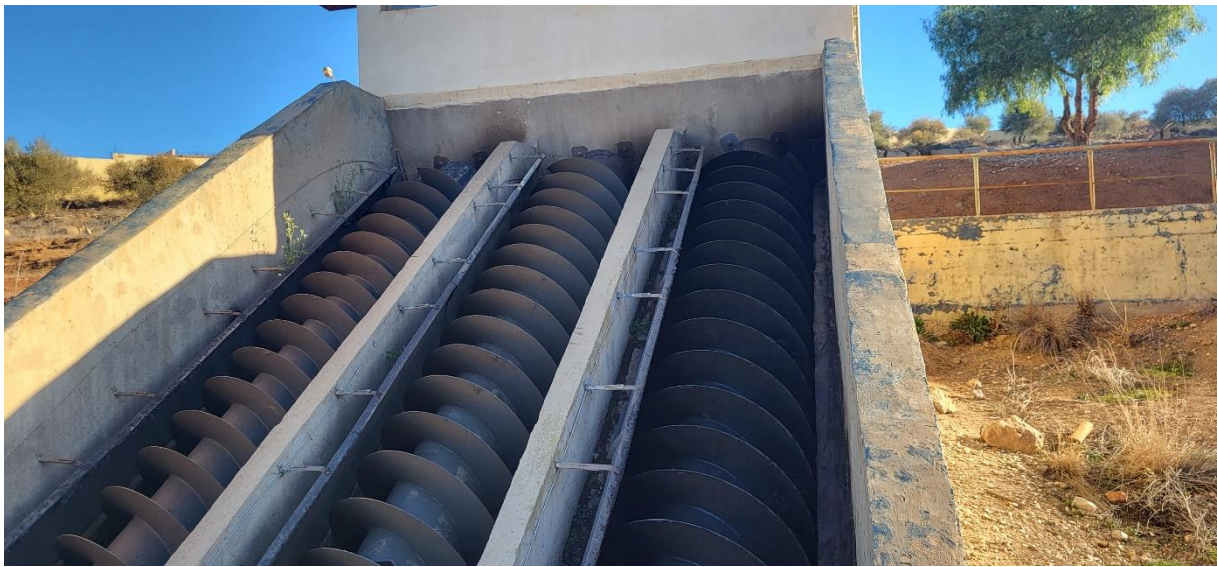
Figure 3. 12 Sludge Pumping Station
