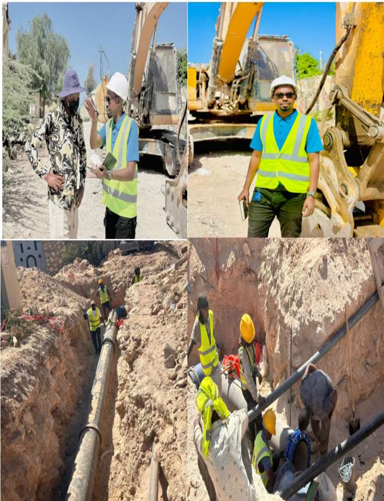
Figure 7: Hargeisa Urban Water Supply Upgrading Project field visit (Photo by the Author, 2024).
