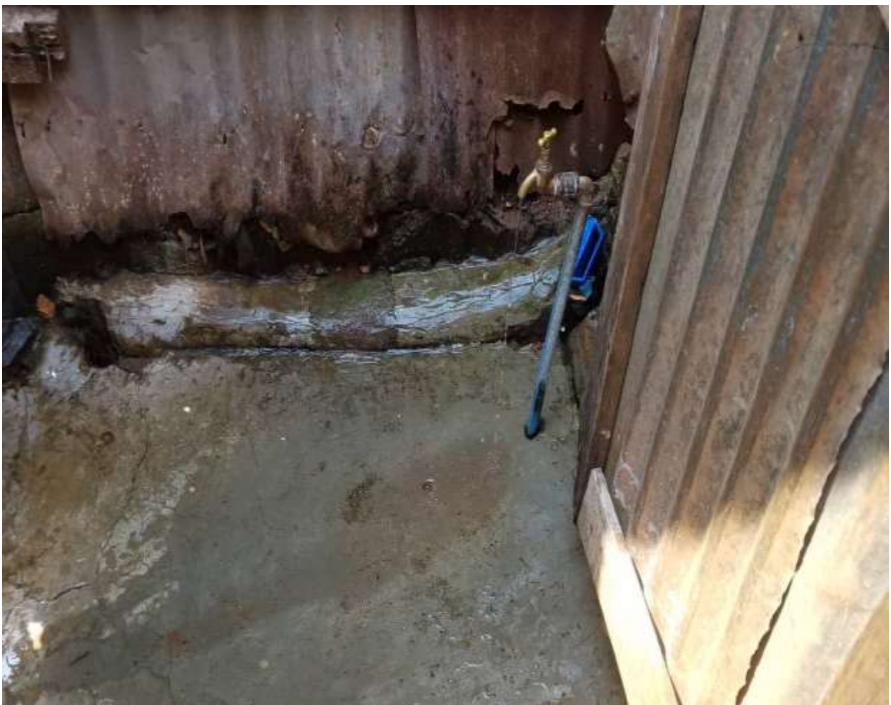
Figure 20: Tap water supply within 100 meters to the households
