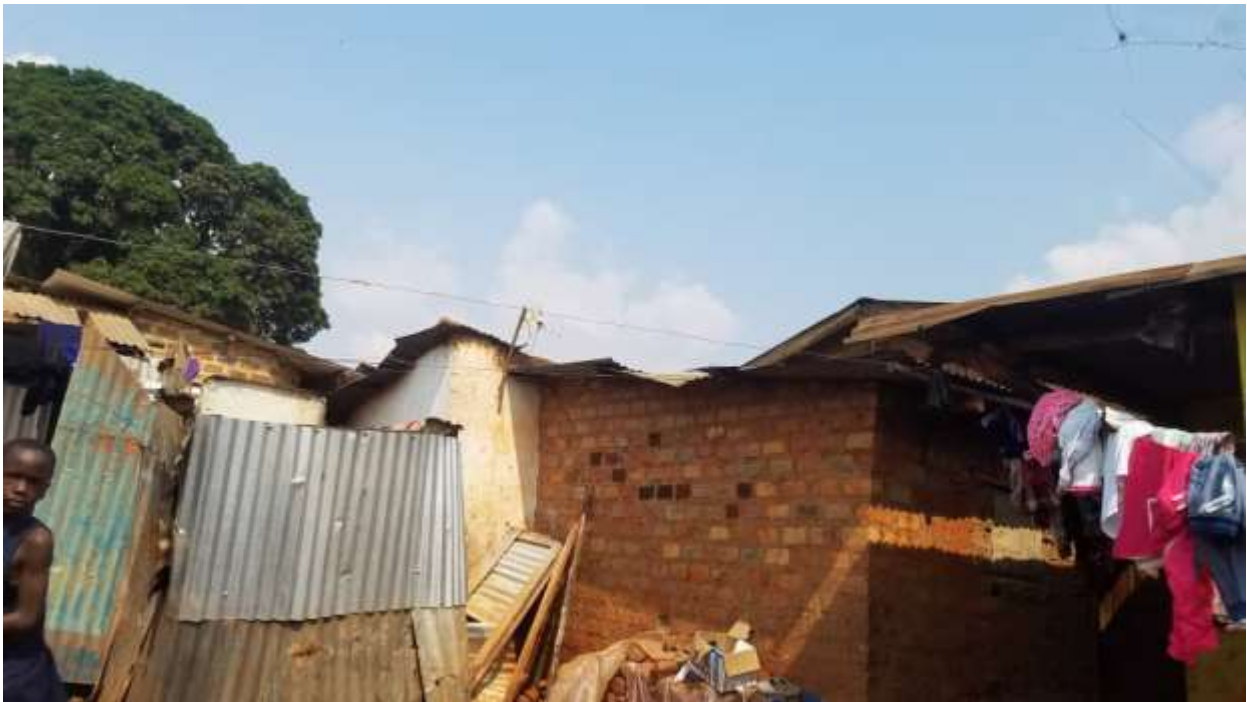
Figure 19: Housing units' conditions in Namatala urban slum
